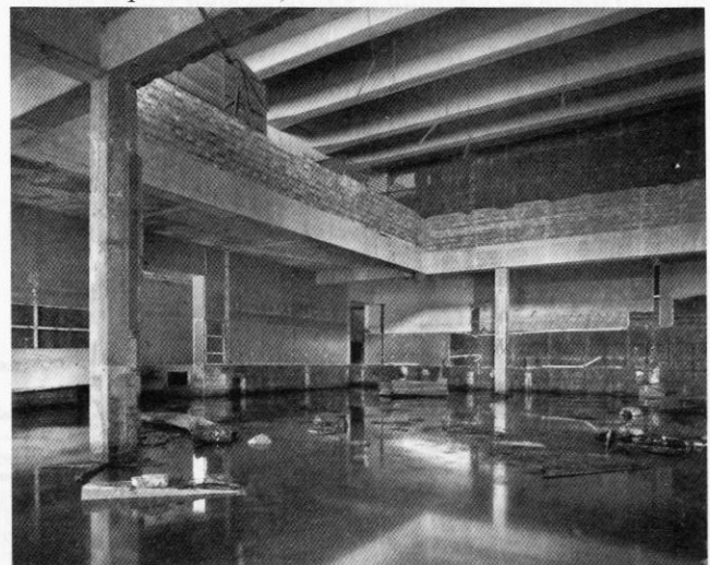
The two level operations room, now stripped of all fixtures and fittings. Photo: Nick Catford
